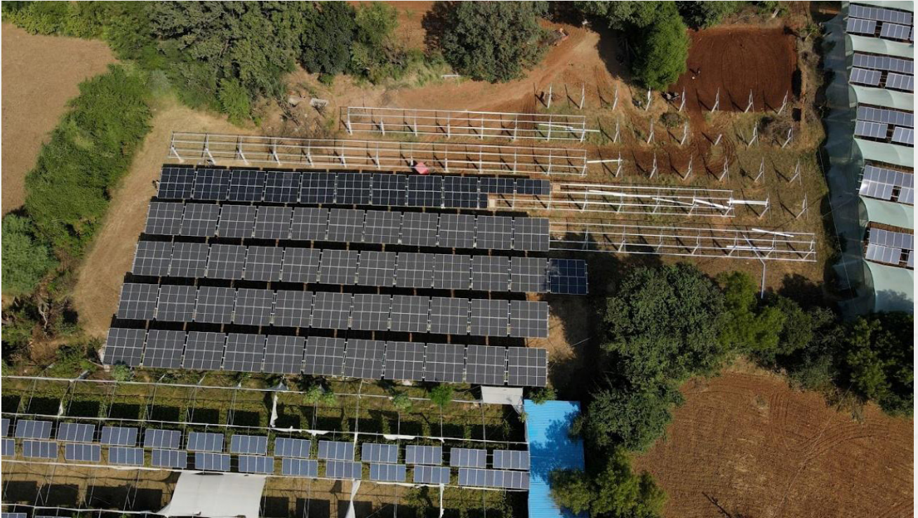
Figure 16. Aerial picture of Indra Solar Farm-2
