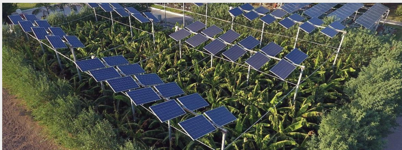
Figure 37. 14.4 kW Agrivoltaics structure with banana (Credit: Jain Irrigation)
